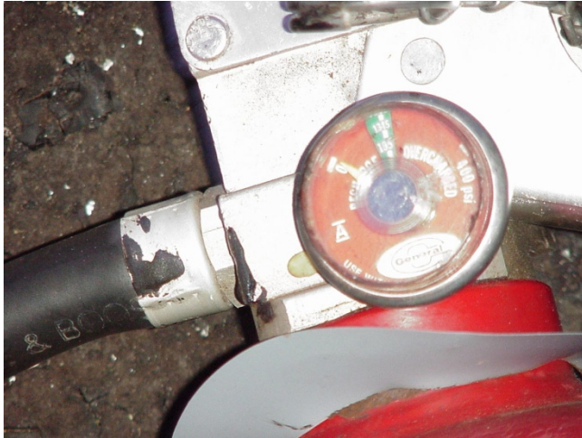
Fire Extinguisher Not Charged
