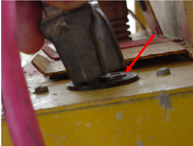
Ground Prong Missing
