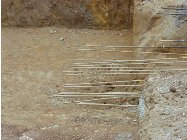
“Rebar” Not Capped
