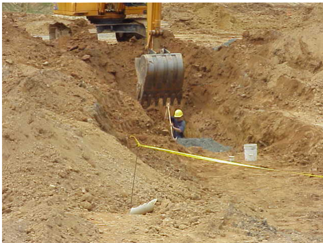
Not properly sloped, benched, etc. Go to “Table of Contents”
