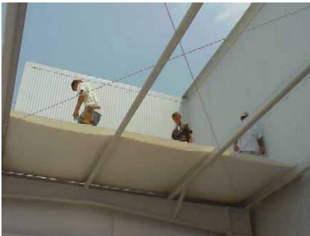
No Fall Protection Equipment Go to "Table of Contents"
