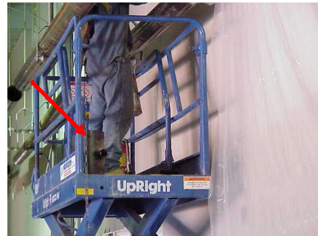
Safety Chain Not Utilized
