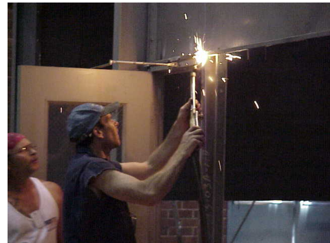
Inadequate Use of PPE
